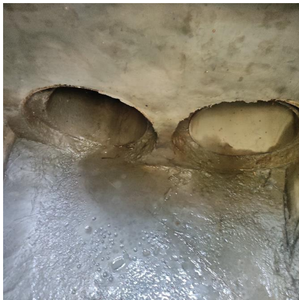
A close-up photograph of a large, circular metal opening, possibly a manhole or access point. The metal is heavily corroded, with a thick, reddish-brown rust layer covering the rim and the surrounding structure. The interior of the opening is dark and appears to be made of a different material, possibly concrete or a smooth metal, showing some signs of wear and discoloration. The lighting is bright, highlighting the texture of the rust and the smooth interior surface.
