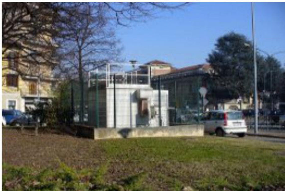
Figura 152. Centralina To – Rebaudengo
